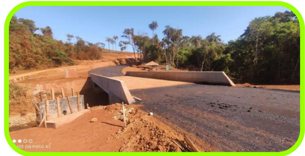
New reinforced bridge over Rio Borrachudo, improving safety and heavy vehicle access.
