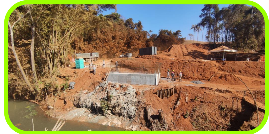
Construction of the reinforced bridge over Rio Borrachudo, enhancing safety and regional connectivity.
